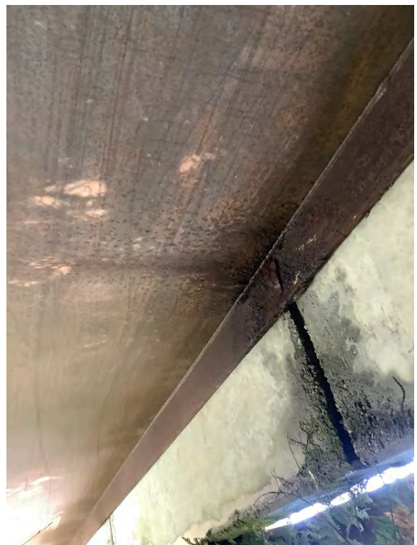
Corrosion Top flange of girder.
